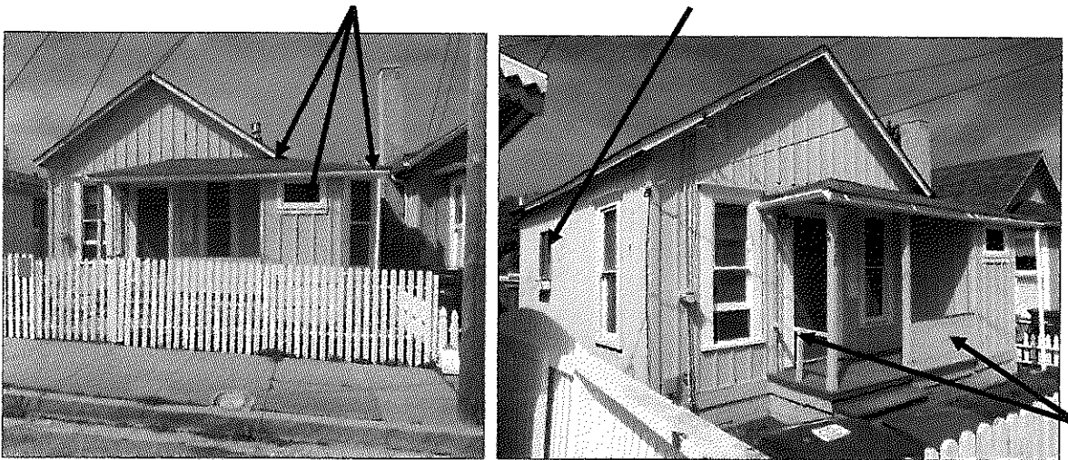
Figures 1 and 2. Left image shows the front (east) elevation, with moving of the north façade wall, porch roof extension, and newer fixed sash window shown with arrows. Right image shows the front (east) and side (south) facades. Porch rails have been replaced (arrows). The newer aluminum slider window is shown with an arrow.
